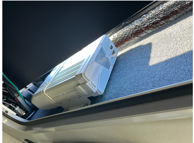
Photo 10 - Representative equipment/configuration view
